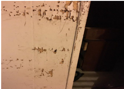
Dining wall paneling-west Risk-nail holes chipped paint
