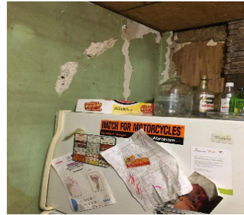
kitchen wall plaster-south Risk-walls scraped, paint dust
