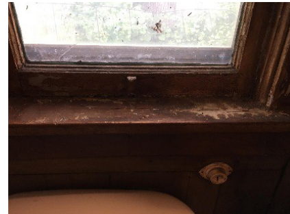
bathroom window-west Risk-chipped woodwork
